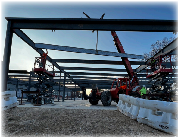
The final steel beam was hoisted into place for Bentonville Public Library’s expansion project on November 17. Photo by Samantha Sacry, Library Marketing Specialist, Bentonville Public Library.
