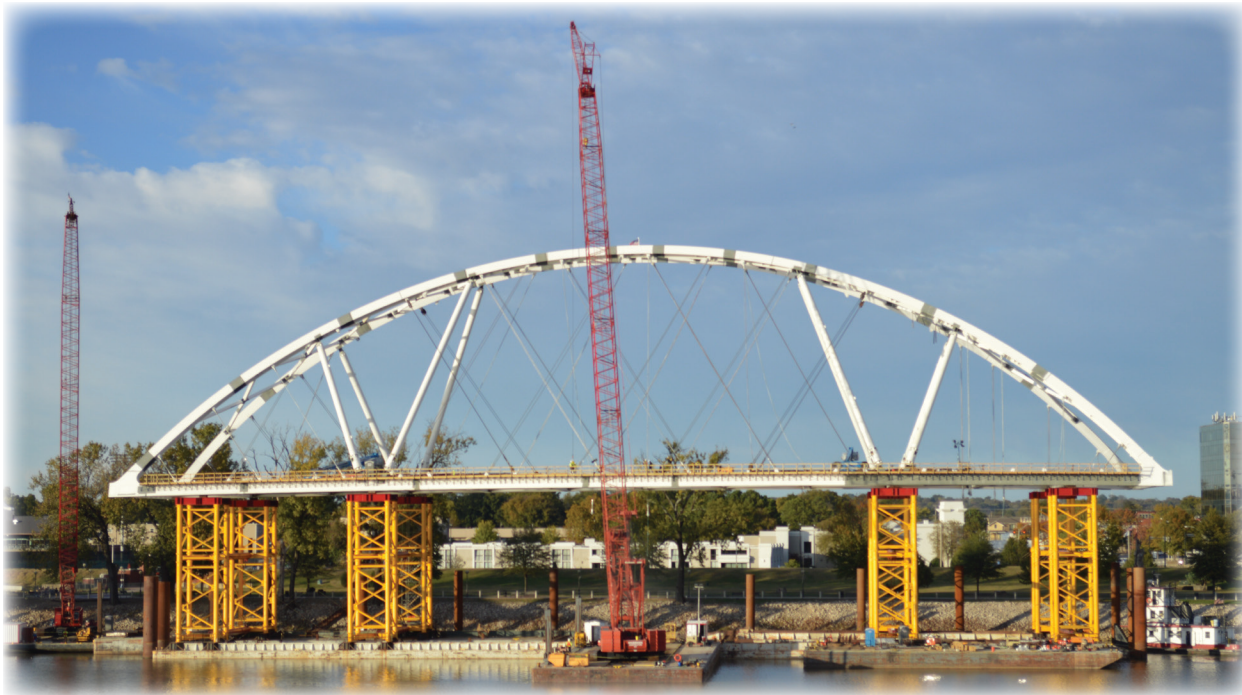
A span of the new Broadway Bridge was put into place as the Conference ended.
